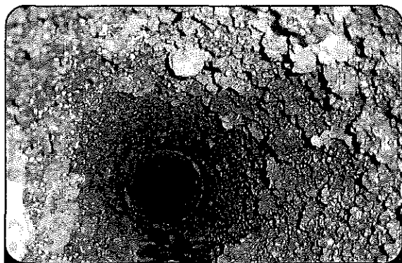
A pipeline prior to line pigging.
